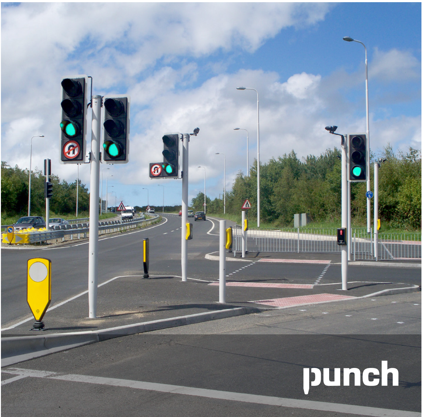
Traffic Signal Poles and push button poles
