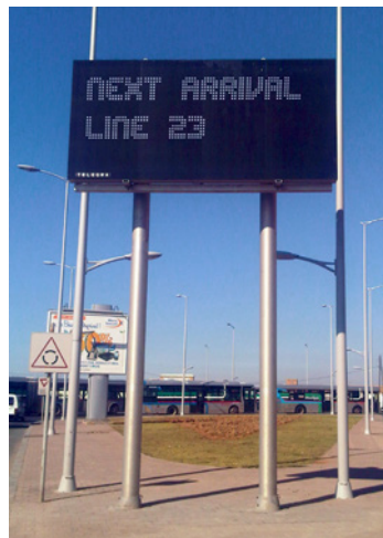
Support for Variable Message Sign
